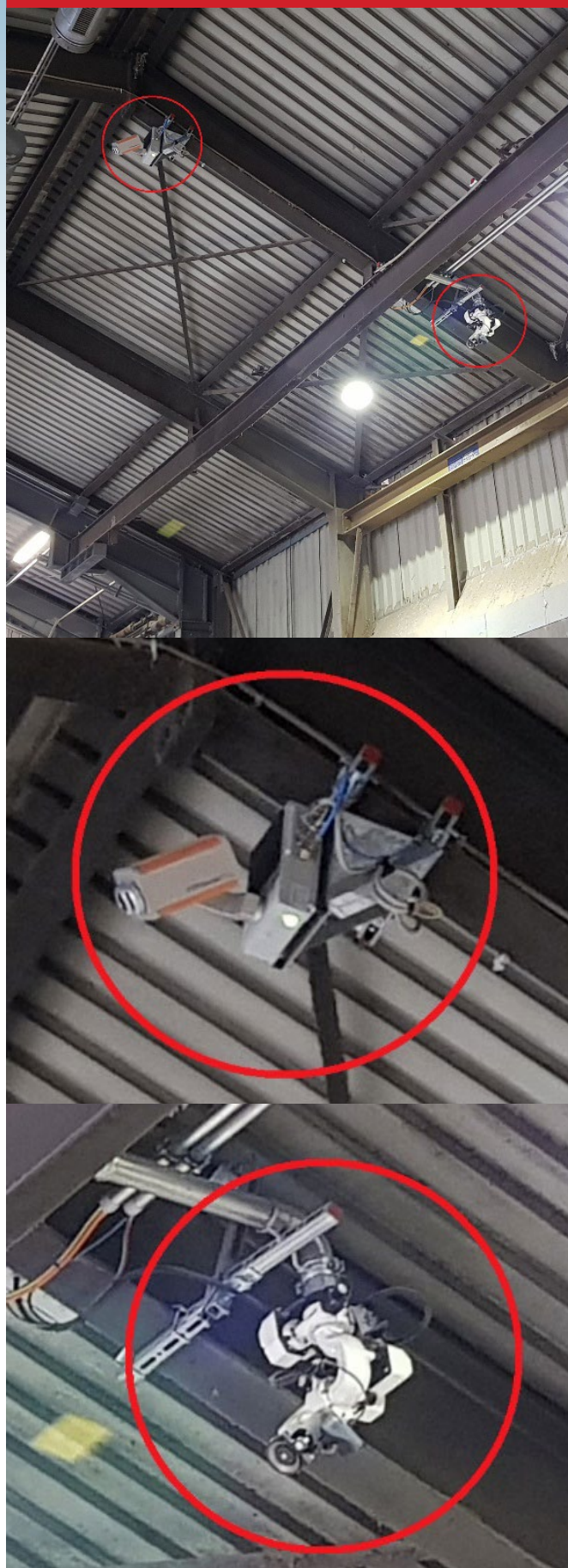
Figure 5 – PYROsmart heat detection system and remote-controlled monitor in recycling plant
